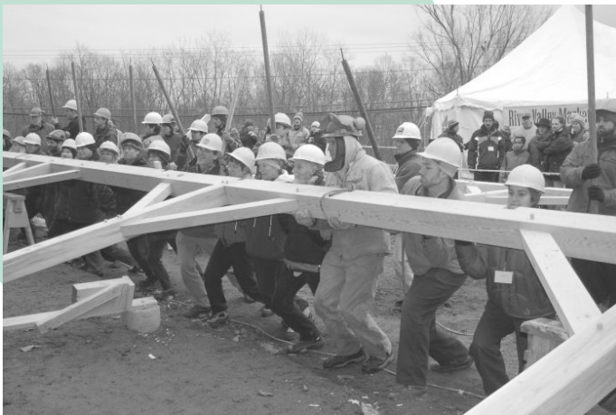
Construction starts at the new River Valley Co-op Market in Northampton, MA. The timbers in the photo were produced by the Massachusetts Woodlands Co-op in S. Deerfield, MA.
