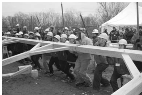
Massachusetts Woodlands Co-op timbers being raised at River Valley Market co-op, Northampton, MA.
